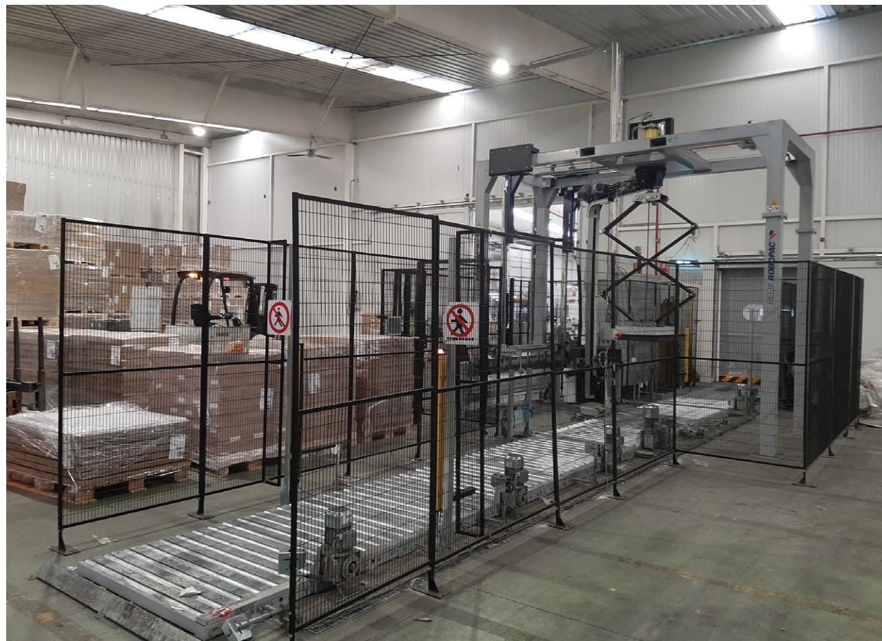
Wrapping machine at the Verescence La Granja finishing plant
